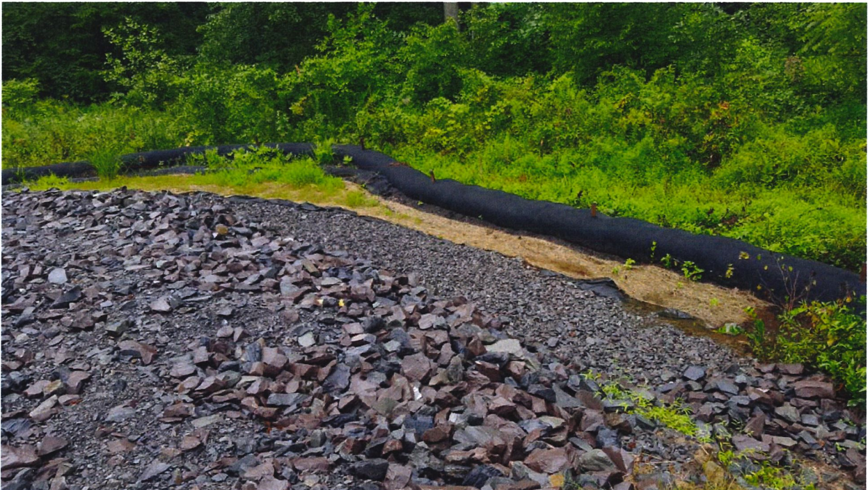
Photo #9: Looking downslope from spillway toward infiltration trench and 24" compost filter sock.
