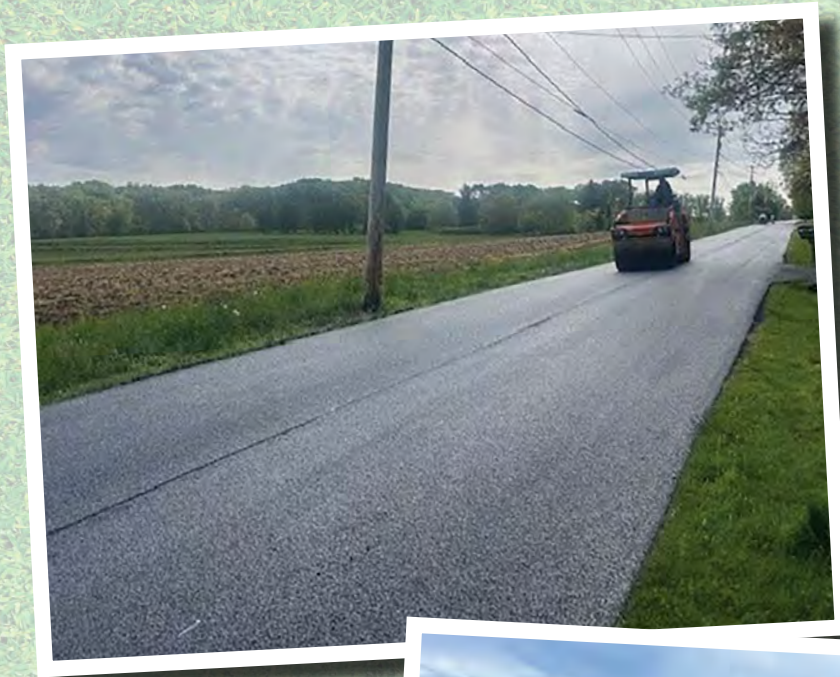
Photo at left: Ultra Thin Bonded Wearing Course on Branch Road and Blooming Glen Road
